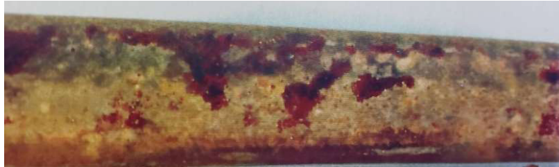
Figure 1. Pipe of steam reheater, after exploitation [8]
