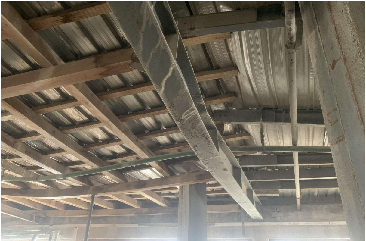
Figure 9. Another position of the wooden and steel section supports plastically deformed sections
