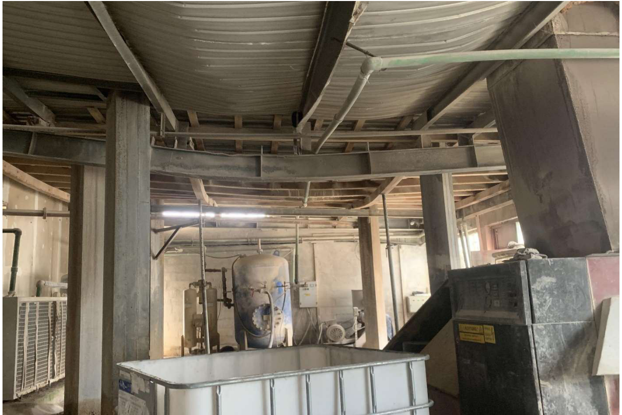
Figure 11. Detailed position of plastically deformed sections & roof
