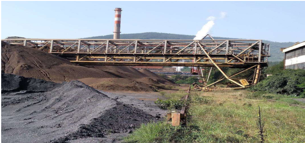
Figure 1. A broken sort of portal crane
