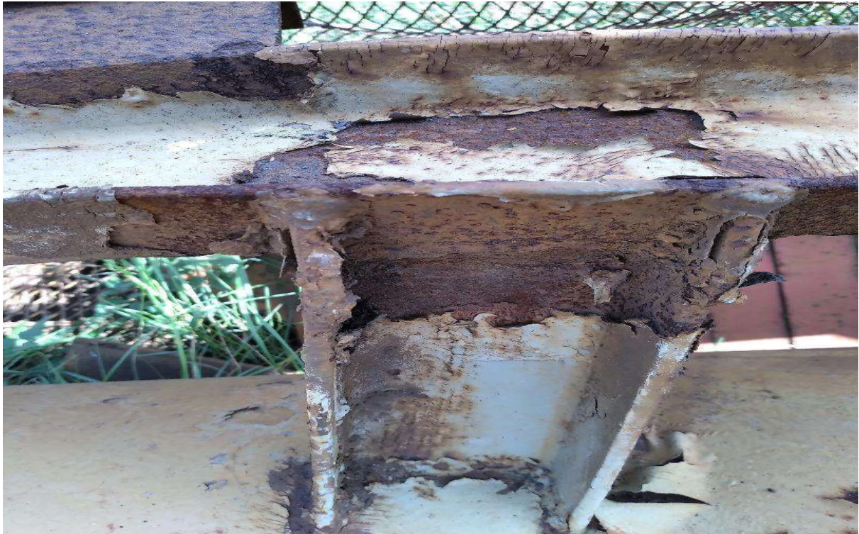
Figure 5. Detailed position of a deeply corroded section of a broken portal crane
