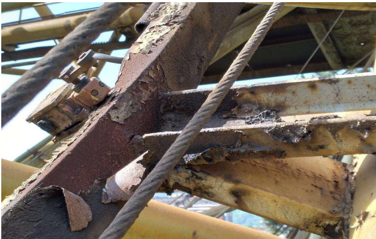
Figure 6. Detailed position of a welded and deeply corroded section of a broken portal crane
