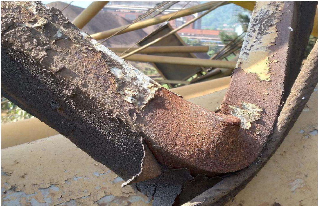
Figure 4. Detailed position of a heavy bended section of a broken portal crane
