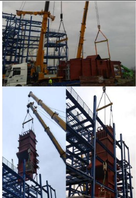
Fig. 4 Attaching the boiler module to cranes, its lifting, rotation and placement in the load-bearing steel structure.
