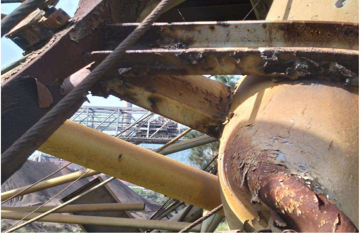
Figure 7. Detailed position of the small ductile breaks of a broken portal crane section
