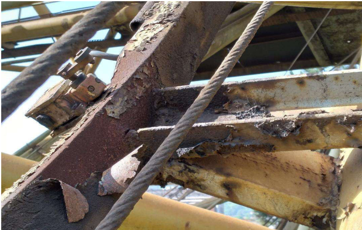
Figure 6. Detailed position of a welded and deeply corroded section of a broken portal crane
