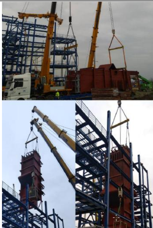
Fig. 4 Attaching the boiler module to cranes, its lifting, rotation and placement in the load-bearing steel structure.
